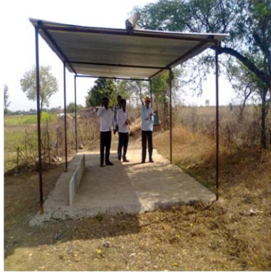
Poorly laid Concrete bed in Methimelkonda, Bidar -Bhalki
