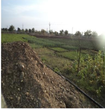
Field bunding built using excavated hard soil of a dug well in Saingaon, Bhalki, Bidar
